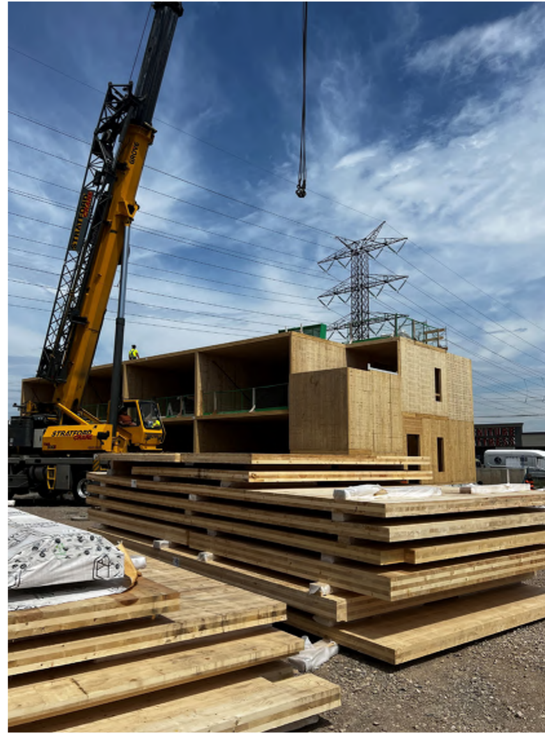
JUNE 13 TH 2024 Superstructure installation up to Second Floor; 3rd week of June anticipated install up to Third Floor with 3-story exterior Wall Panels.
